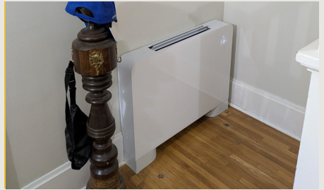
Fan coil with room-by-room thermostat.
