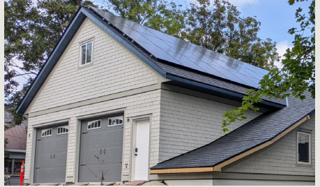
Solar panels on new garage roof.
